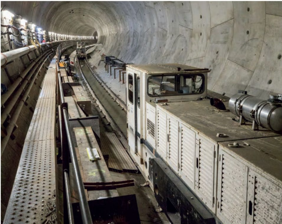
The existing surface will be covered by an in-situ poured concrete lining PHOTO: ABSOLUTE PHOTOGRAPHY LTD
